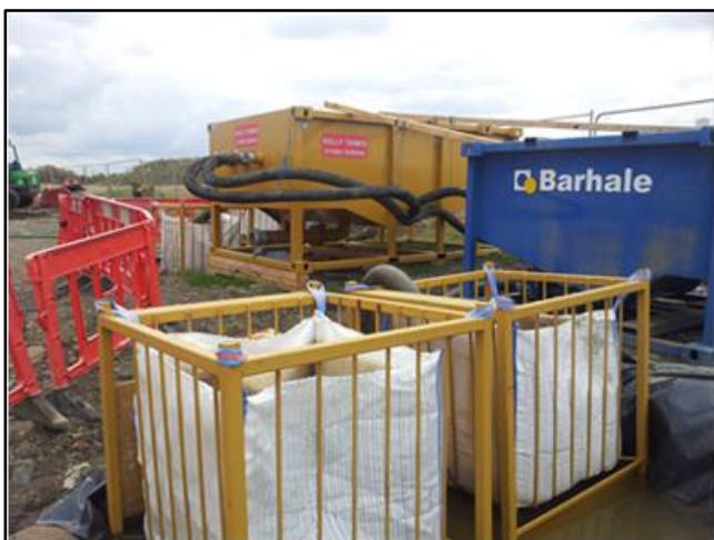
Groundwater treatment System
